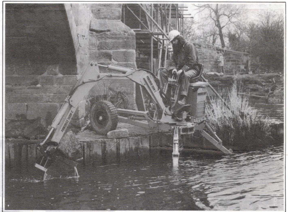
Half-in and half-out of the water, the Powerfab climbing excavator digs out debris from the bridge piers.
